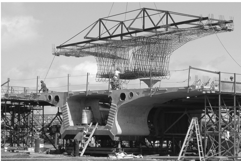
Fig. 3. Match casting, where each new segment is cast against the previously completed one to ensure that all the pieces fit together properly. The curved shape of segments was one of the bridge's aesthetic features.
